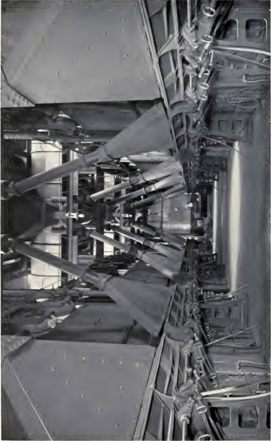
POTOMAC ELECTRIC CO., WASHINGTON, D. C. BABCOCK & WILCOX SUPERHEATERS INSTALLED IN 12,000 HORSE POWER OF BABCOCK & WILCOX BOILERS
